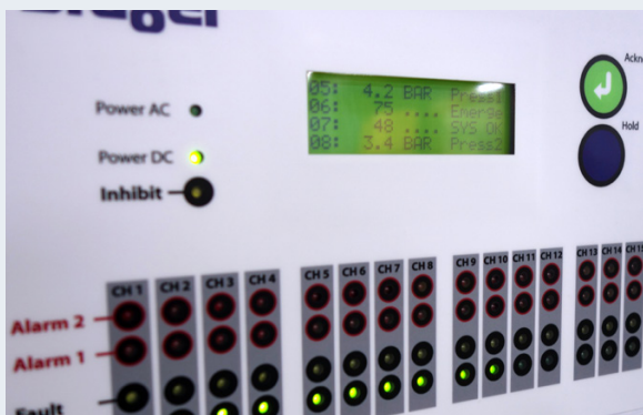
SAFETY CONTROL SYSTEMS PLC
